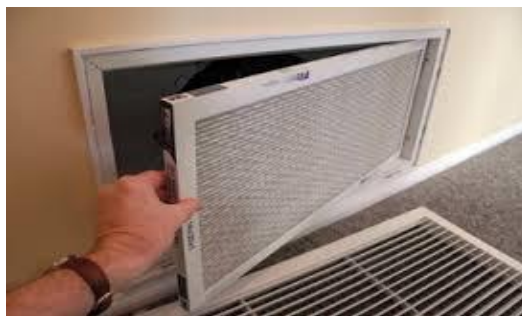
Filter in wall
