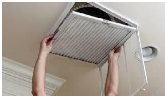
Filter in ceiling
