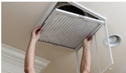
Filter in ceiling
