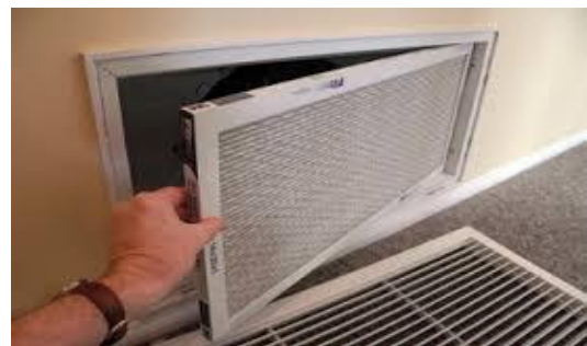
Filter in wall
