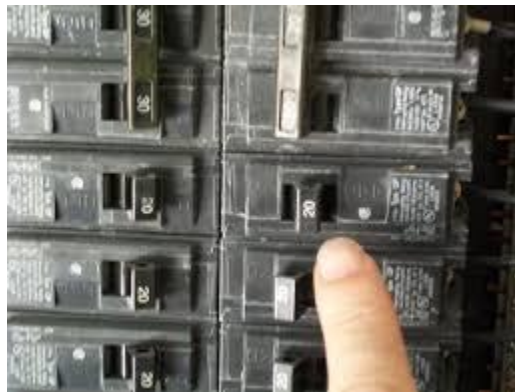
Reset Circuit Breakers
